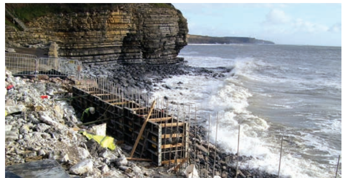
Construction of sea defences form a major part of works in the South West
