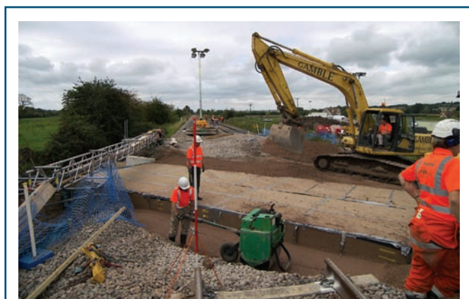
RAIL CULVERTS REPLACED: Two collapsed culverts in Berkshire passing beneath railway near Reading were replaced during a 52 hour blockade of lines in September. The works (pictured above) preceded the repair and treatment of two bridges in south Wales which formed part of the same contract on behalf of Network Rail. The £812,000 'Four structures' package includes replacing Midgham Culvert near Newbury and the Quarry Tunnel Bridge in south Wales. The contract is expected to be completed in June.
